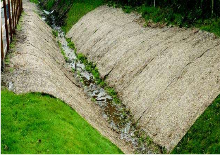
Figure 10-4 - Erosion Control Blanket
